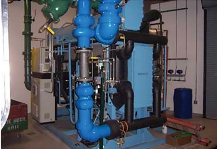
A 300-ton absorption chiller located at a data and research center at Syracuse University, New York. The chiller uses exhaust from twelve 65-kW microturbines and can cool water to 45°F. Photo courtesy of New York-New Jersey Onsite Energy Technical Assistance Partnership (TAP).
