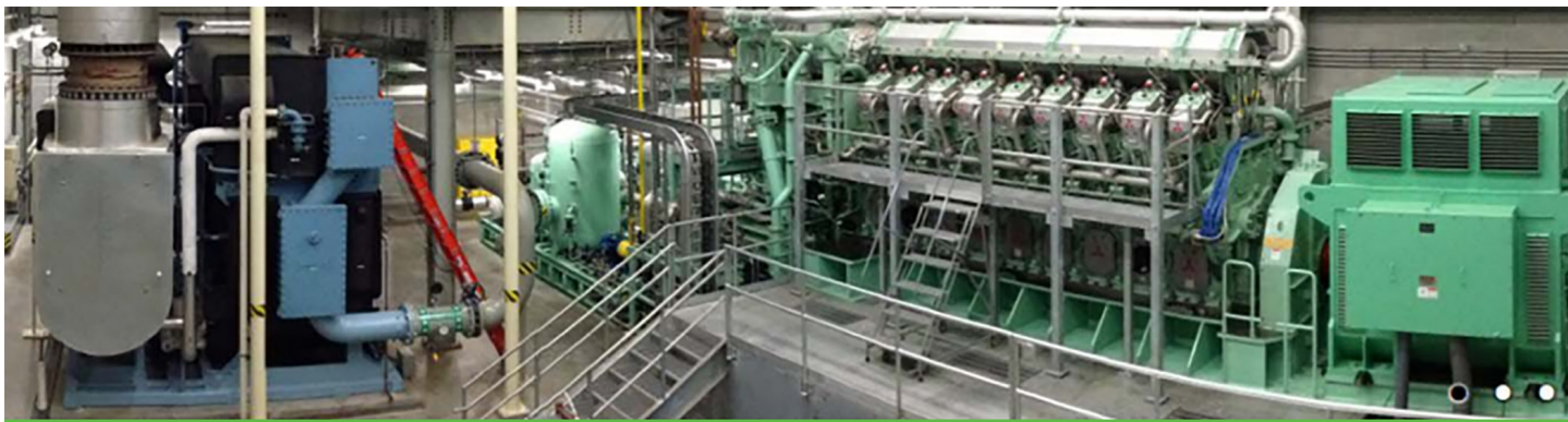
A 992-ton absorption chiller (left) integrated with a reciprocating engine at the University of Central Florida. The chiller is used to supplement the district chilled water system and uses waste heat and exhaust from the engine (right). Photo courtesy of the Southcentral Onsite Energy Technical Assistance Partnership (TAP).
